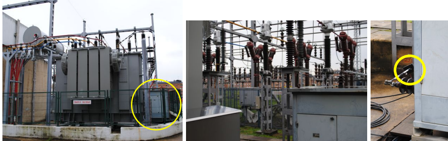
Fig. 1. La Corredoria substation transformer and its NGR (left part). Detail of the connection between the NGR and the neutral (center) and ground (right), showing the current transformer used in this paper.
